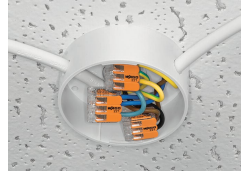
Lighting distribution in a ceiling canopy
