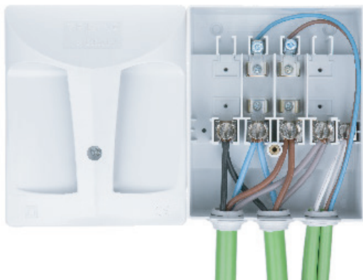
Example of connection inside a box
